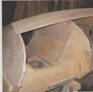
8 The transom, frames and bulkheads are pre-cut to receive each plank. Note how the aft bulkhead is attached to the jig, to hold it square.
