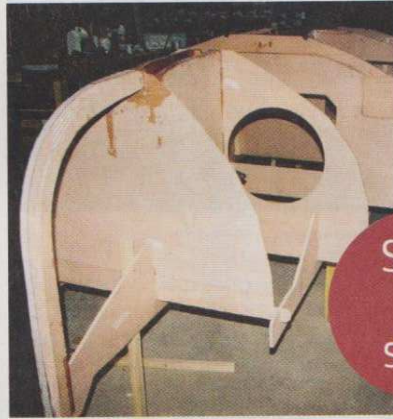
5 Once complete and cured the inner stem is epoxied to the forward bulkhead, the jig holding everything correctly in line.
