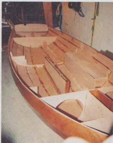
19 Planking complete, the hull can be detached from the jig and turned over to reveal the developing boat.
